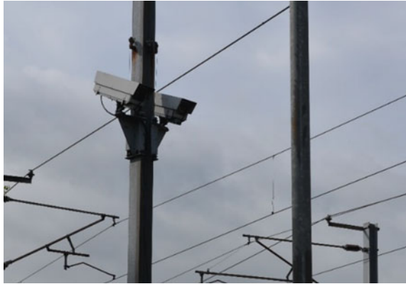
Fig. 9 CCTV camera monitoring Cromwell Lane level crossing
