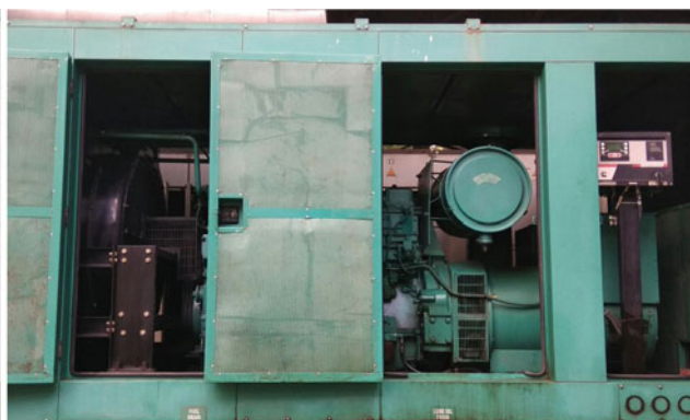
Diesel engine generator
