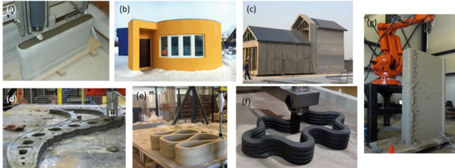
Fig. 65.1 Examples of 3D concrete printing: (a) counter crafting, USA; (b) Apis Cor, Russia; (c) Winsun, China; (d) Loughborough University, UK; (e) TU/e, Netherlands; (f) NTU, Singapore; (g) CyBe
