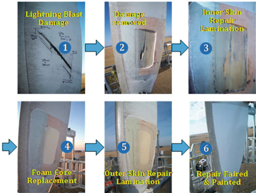
Fig. 8.5 An example of current structural repairing. (Courtesy of Performance Composite Inc. (Performance Composite Inc. 2015))
