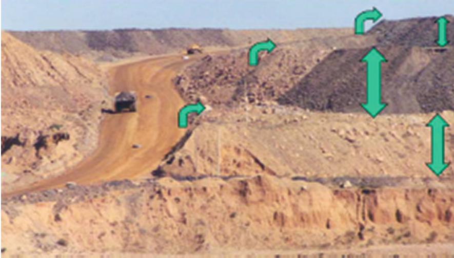
Fig. 2.10 Free dumping is seen in form of compressed lifts in an opencast mine [16]
