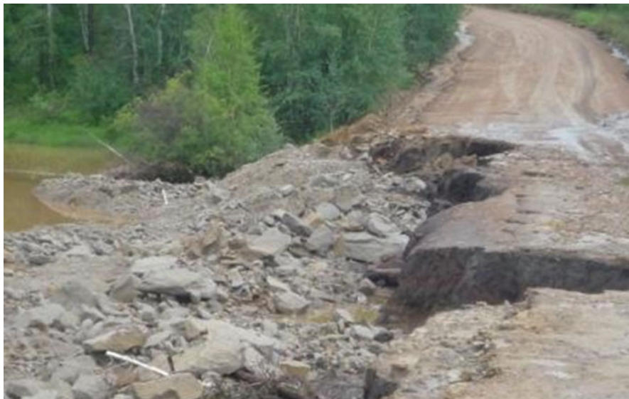
Fig. 14.4 Catastrophic mudflow after heavy rains closed the highway Yakutsk-Amga. (Photo of July 2013 [3])
