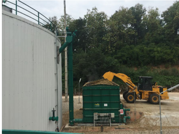
Fig. 3.18 Combination of horizontal, vertical, and inclined screw conveyors to transport the material from a solid feeder to a digester
