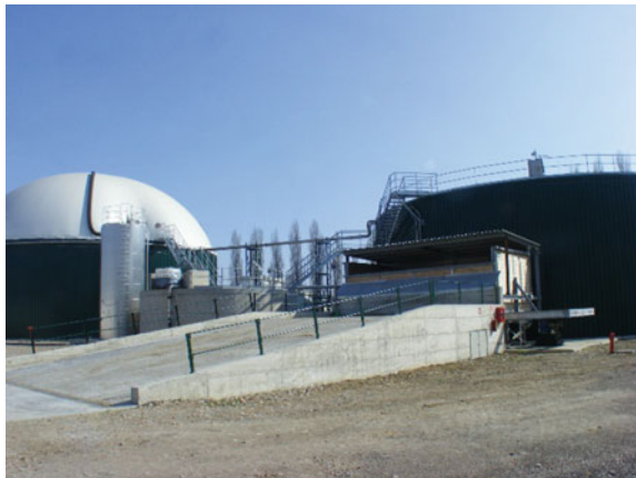
Fig. 3.15 Wood wall solid feeder installed on Sebigas a division of Exergy S.p.A. plant
