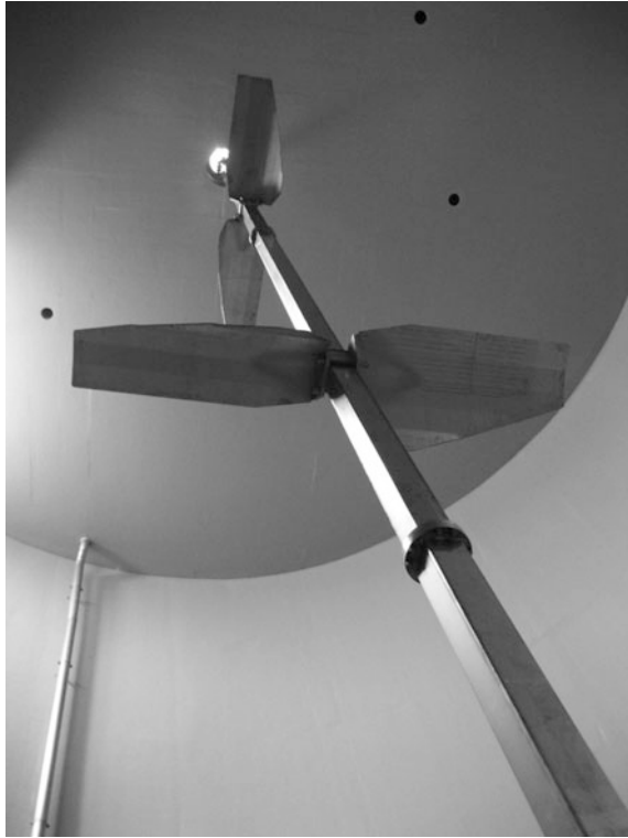
Fig. 3.28 Vertical shaft slow speed agitator installed at the centre of the digester roof [Stamo Maskin AB]
