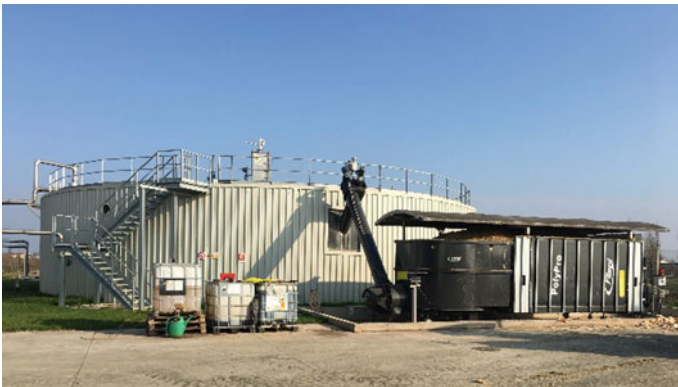
Fig. 3.19 Example of an inclined screw conveyor to transport the materials from a solid feeder to a digester [Sebigas a division of Exergy S.p.A.]
