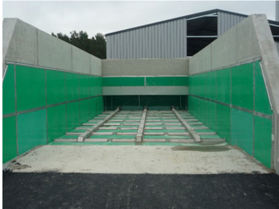
Fig. 3.11 Example of push floor rack installed in concrete bunker with lining protection from corrosion [Huning Anlagenbau GmbH & Co. KG]
