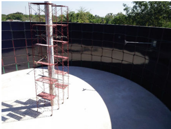
Fig. 3.27 Inclined mixer with external motor during installation [Sebigas UAC Co., Ltd.]
