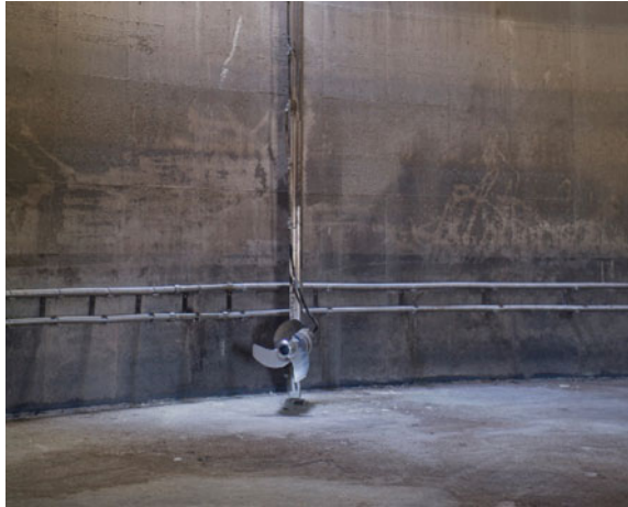
Fig. 3.25 Submersible mixer installed in concrete tank digester
