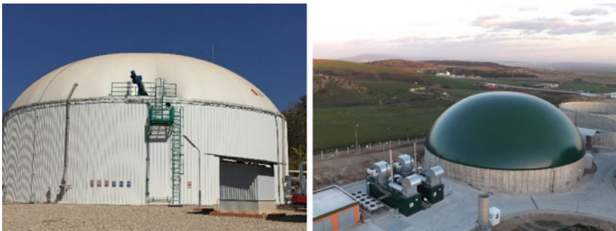
Fig. 3.30 Example of PVC-coated fabric gasholder installed
