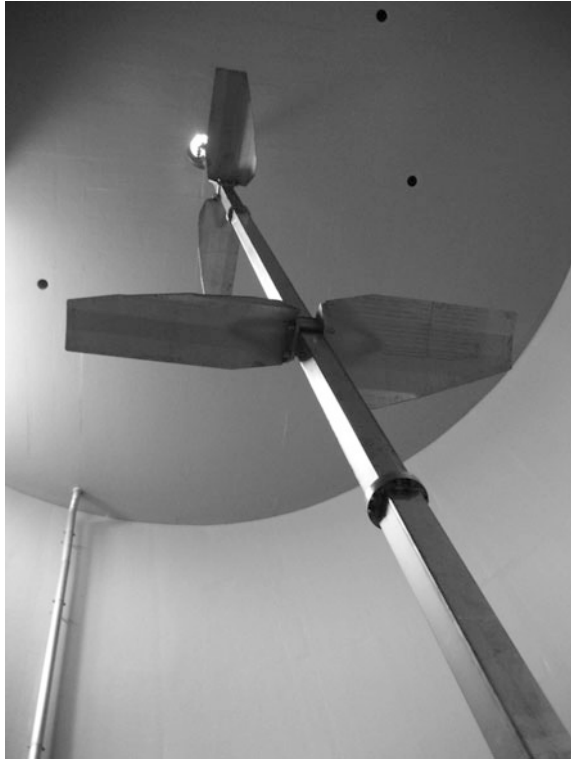
Fig. 3.28 Vertical shaft slow speed agitator installed at the centre of the digester roof [Stamo Maskin AB]
