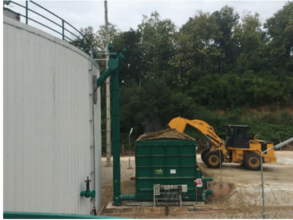
Fig. 3.18 Combination of horizontal, vertical, and inclined screw conveyors to transport the material from a solid feeder to a digester
