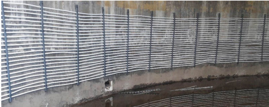
Fig. 8.2 Internal loop (warm water) for heating the digester
