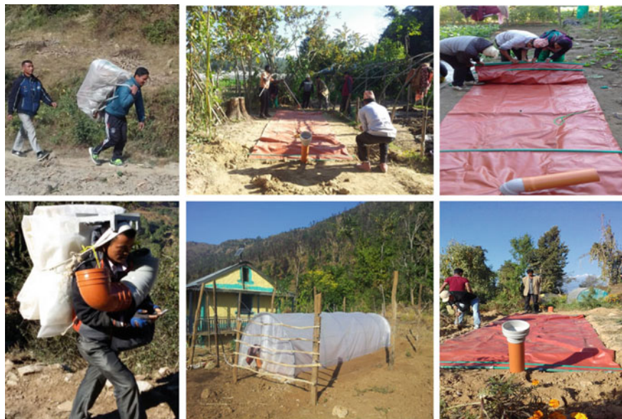
Fig. 18.4 Portable biogas installation in the hilly areas of Nepal
