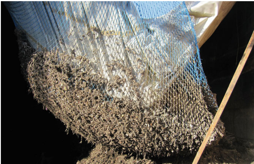
Fig. 8.11 Scum formation and its penetration into the inner cover layer of the digester
