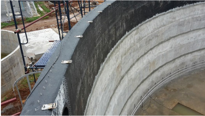
Fig. 3.24 PE membrane protection installed during pouring of the concrete to protect the surface above liquid level
