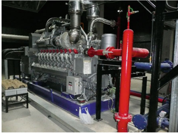
Fig. 3.31 MTU biogas engine installed in power-house solution [MSM Energy Solutions Co., Ltd.]
