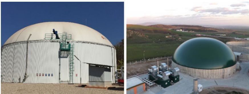
Fig. 3.30 Example of PVC-coated fabric gasholder installed
