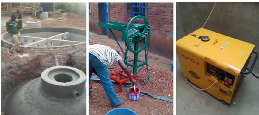
Fig. 18.5 Installation of a 48 m 3 digester at a communal cow shed in Rwanda
