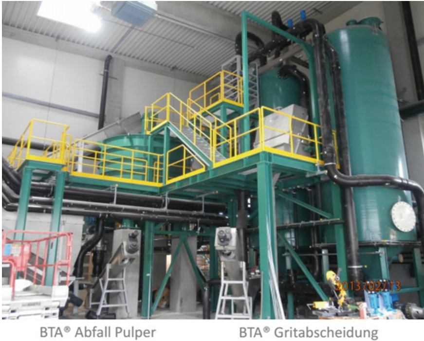
Fig. 5.7 BTA-plant Zell am See, Austria Courtesy BTA-International Co. (Kübler et al. 2015)
