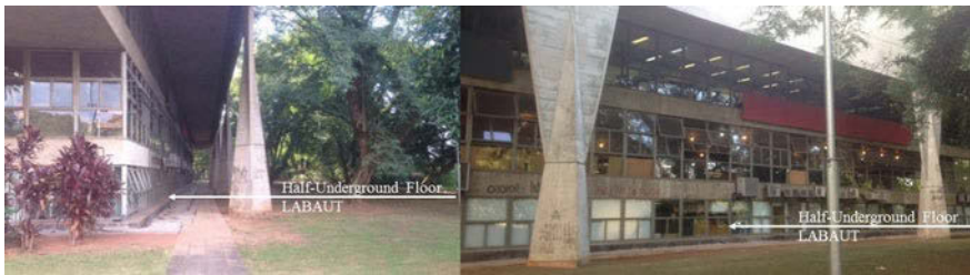
Fig. 6 Views of the concrete wall supported by the trapezoids shaped columns; indication of the LABAUT at the half-underground floor. Source Images from the authors
