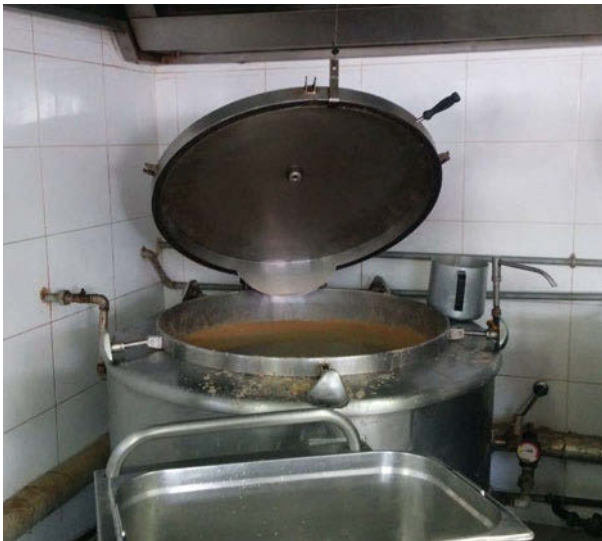
Fig. 2 Picture of one of the restaurant's industrial pans
