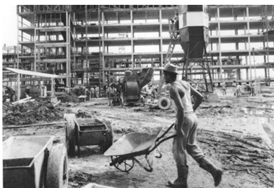
Fig. 2 Construction of the campus' student residences. "Construção do CRUSP". Acervo Digital da USP, accessed August 3, 2017, http://200.144.182.66/acervo/items/show/205
