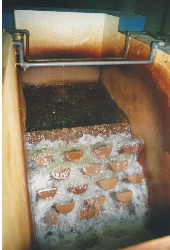
Fig. 6 Dosing of ferric chloride in a cascade
