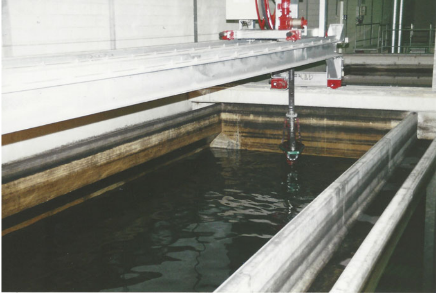
Fig. 12 GAC filter at Leiden (the Netherlands)
