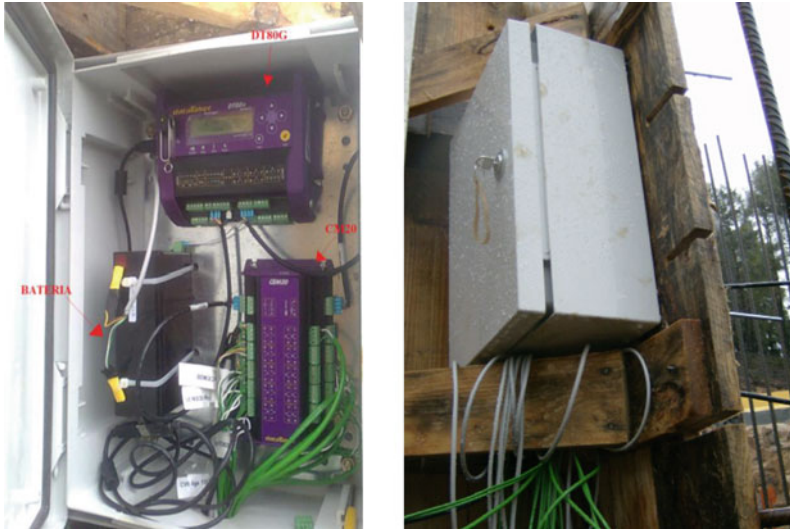
(a) Data logger and battery inside the box (b) Impermeable electric box with data logger inside
