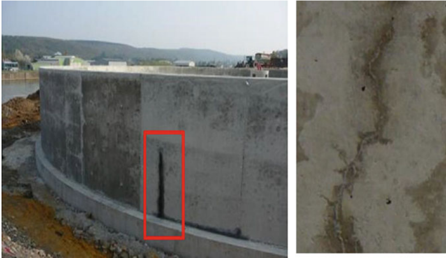
Fig. 8.4 Water treatment plant showing cracking due to the restrained shrinkage at early age and some self-healed cracks (photograph: A. Darquennes)
