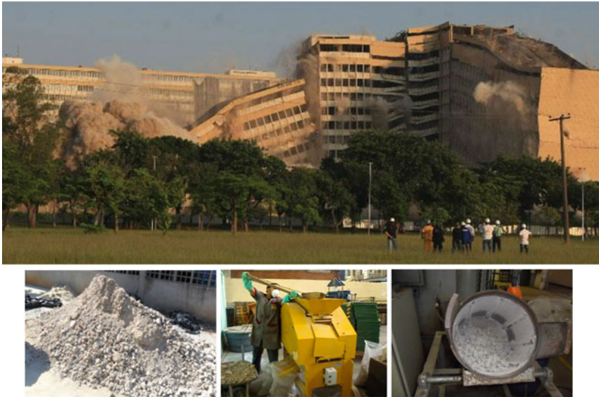
Fig. 10.3 (Up) Demolition of hospital section, Ilha do Fundão, Rio de Janeiro, Brazil; (down left to right) homogenization process, grinding process with a crusher and autogenous cleaning
