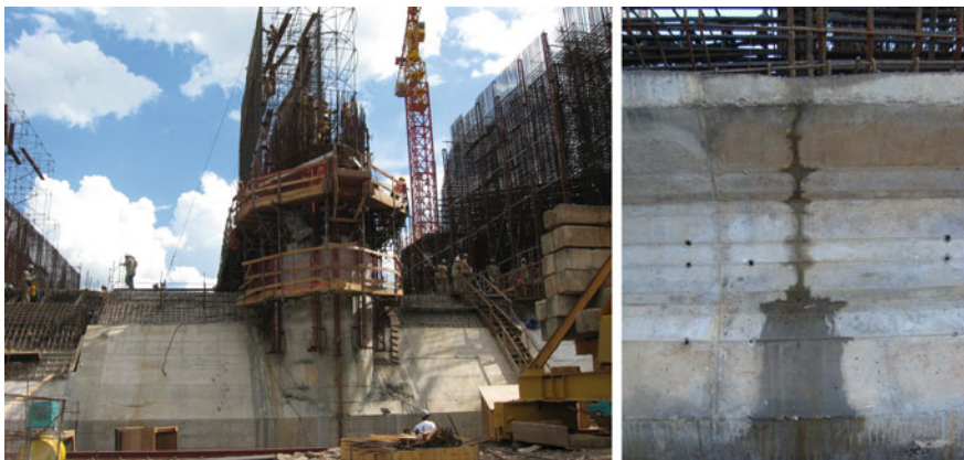
Fig. 1.4 Spillway of small hydropower plant and thermal cracking (Funahashi and Kuperman 2010)
