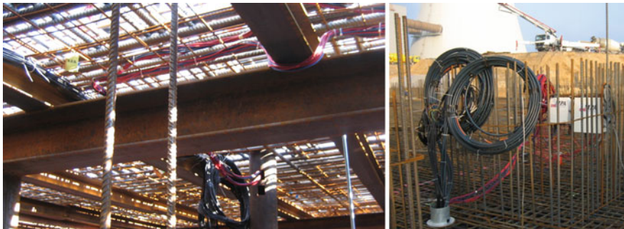
Fig. 9.4 Cable routing and arrangement of the data logger in the monitoring programme of the 4.0-m-thick power plant slab Boxberg (Photos D. Schlicke)
