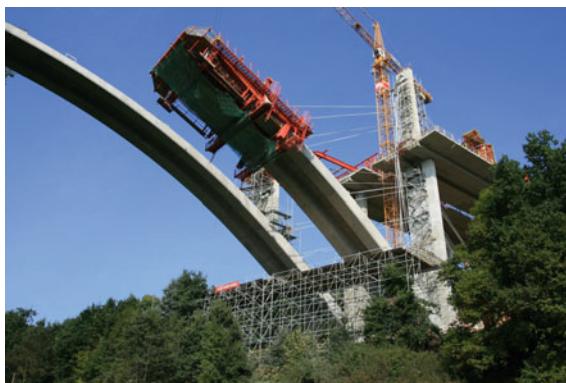
Fig. 7.6 Two arches of Oparno Bridge during construction (Photograph by Jan L. Vitek)
