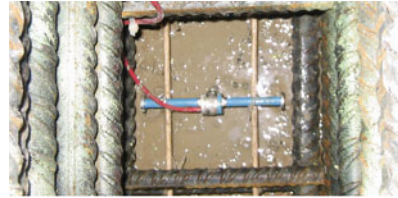
(b) vibrating wire sensor applied in the reinforcement layer (photo: D. Schlicke)
