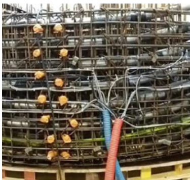
(a) sensor and their cables distributed in the circumference of the vessel
