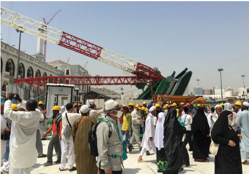
Fig. 11.2 A collapse of construction crane over Mecca's Grand Mosque causing dozens of victims (the authors)
