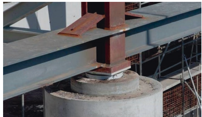
Fig. 26 Detail of the structural support of the main building's external wall under construction
