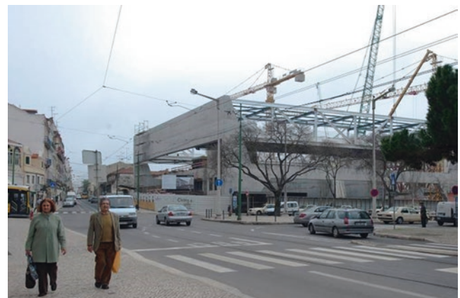
Fig. 22 Street view of the auditorium from Junqueira Street under structural construction phase
