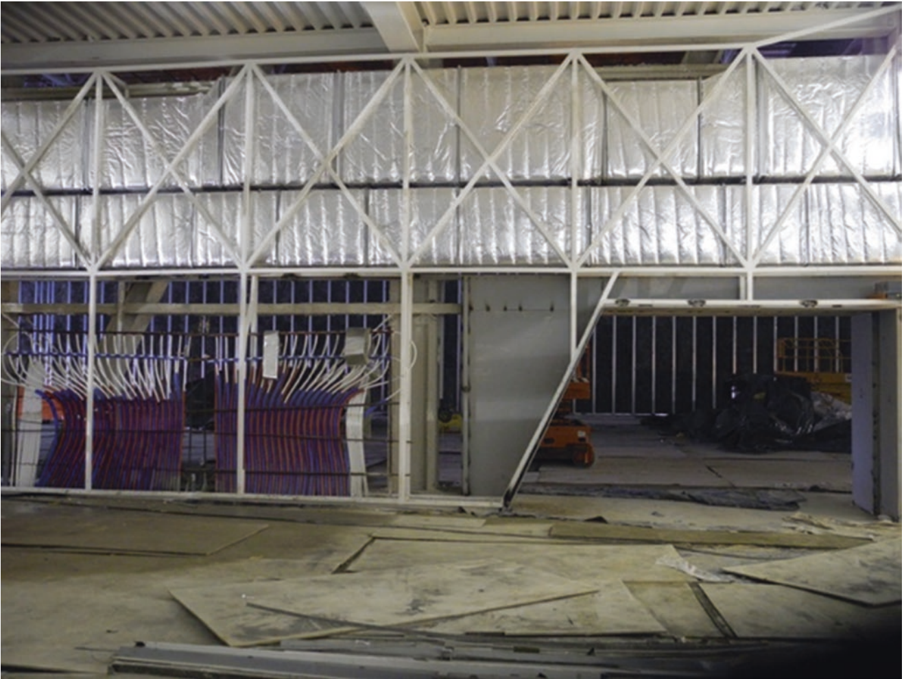
Fig. 90 Ventilation system inside the main wall
