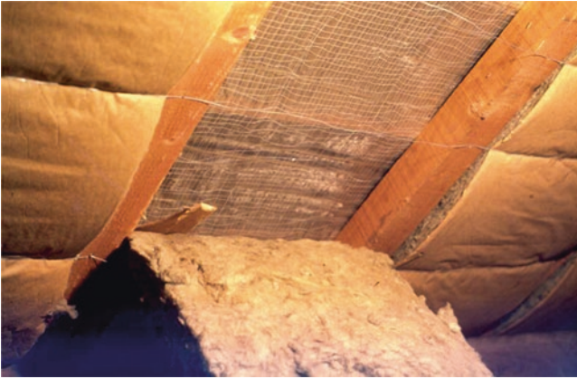
Fig. 5 Insulated pitched roofs, leaky vapour retarder and vapour-tight, non-capillary underlay. The result is an interstitial condensation deposit with run-off and water leakage at the roof edges
