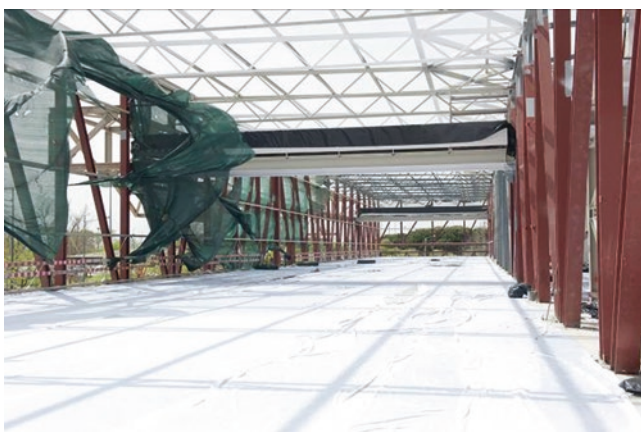
Fig. 12 View of the main room of the museum in the structural construction phase
