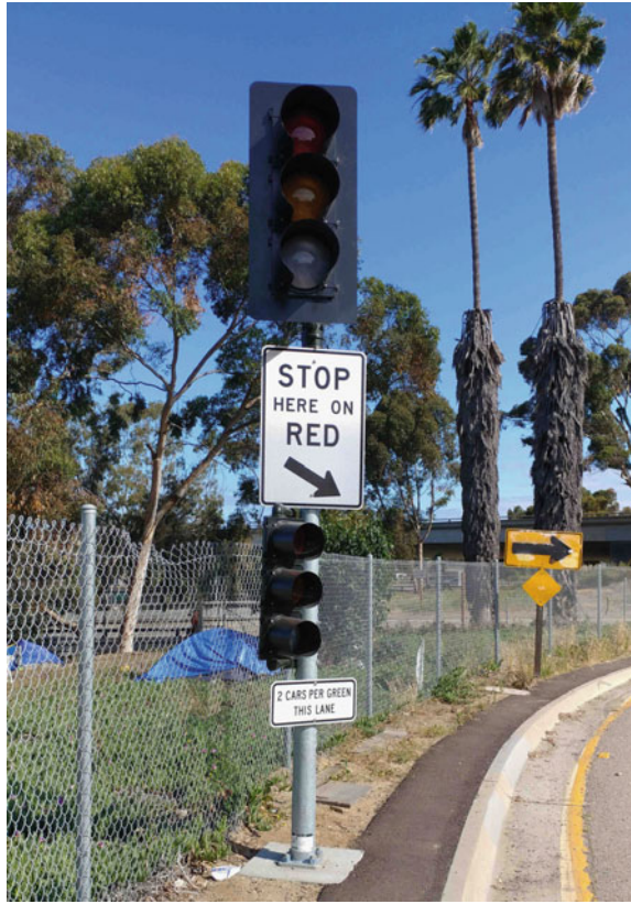
Fig. 1.9 A ramp metering installation in downtown San Diego to State Highway 94, U.S. (courtesy of Michael Ballard)
