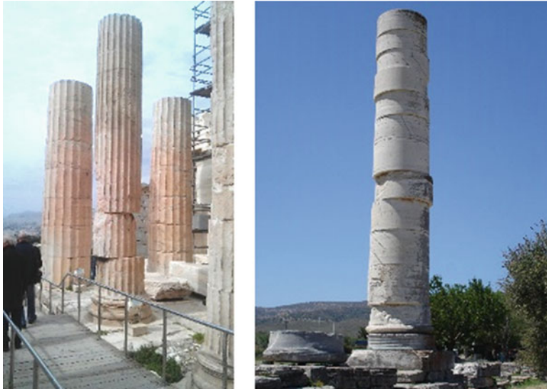
Fig. 24.9 Classical columns with significant drum dislocations. Left: Columns at Propylaea of the Acropolis of Athens, Greece; Right: Column of the temple of Hera in Samos, Greece
