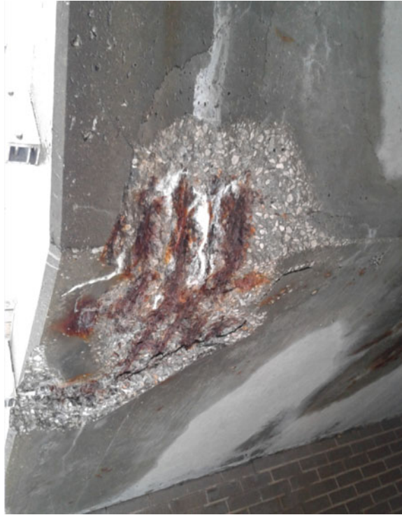
Fig. 1 Corroded rebar under concrete slab
