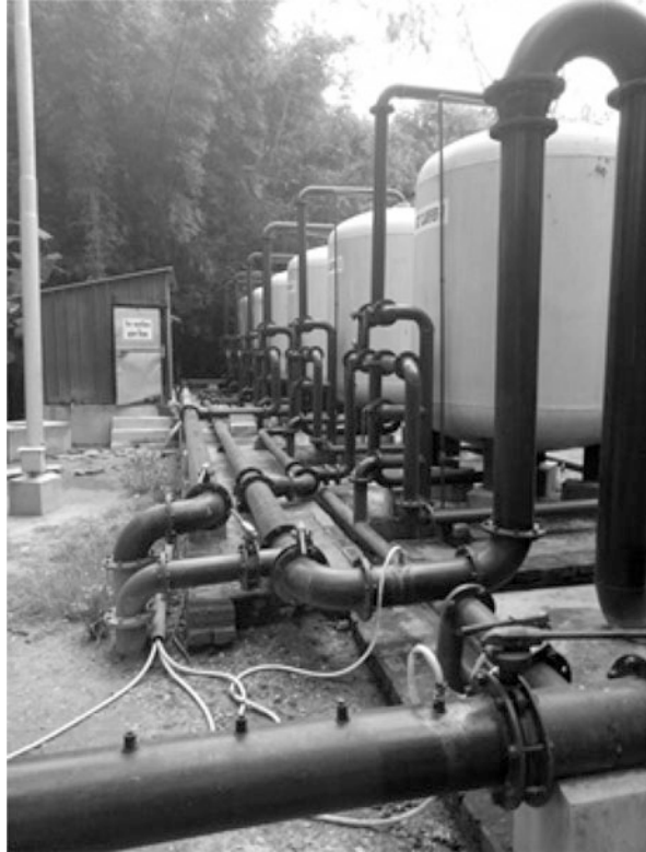
Fig. 16.6 Jasaikathi arsenic and iron removal plant
