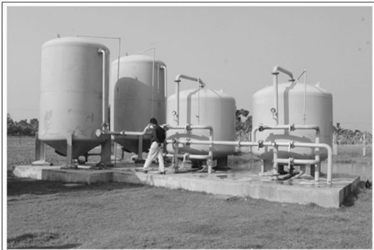
Fig. 16.9 Kola arsenic and iron removal plant
