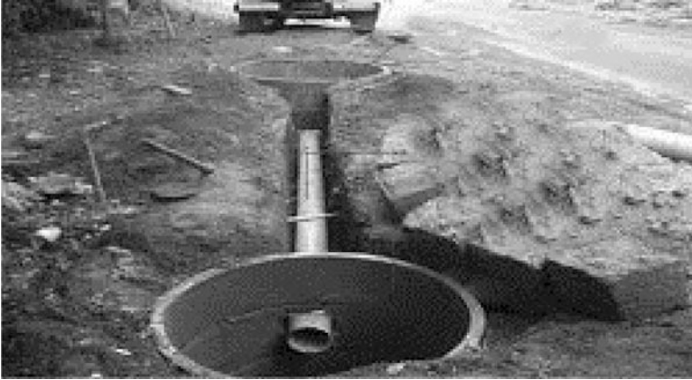
Fig. 18.1 Rainwater harvesting through dug well
