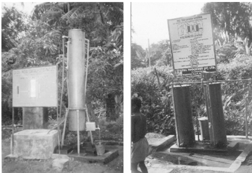
Fig. 16.3 Arsenic removal unit operated with adsorption process
