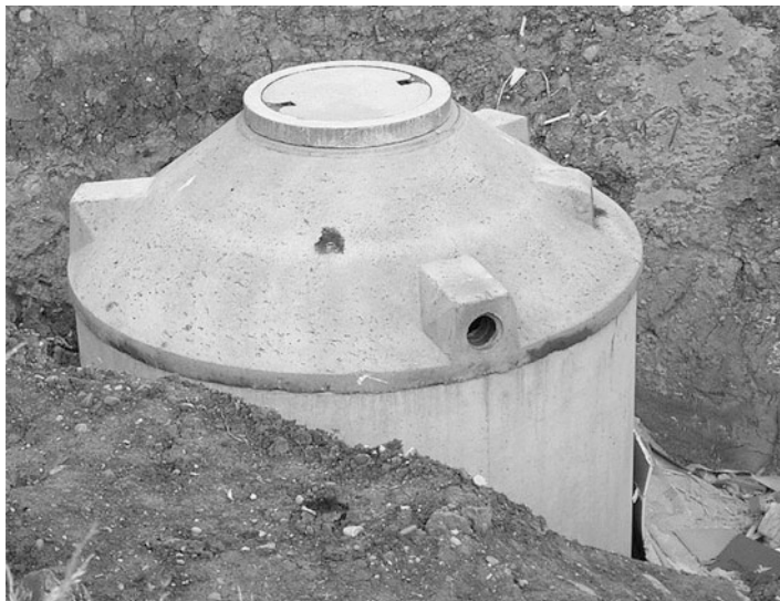
Fig. 18.5 A rainwater collector tank
