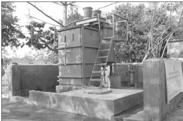
Fig. 16.5 Arsenic removal unit operated with two-stage treatment at Malatipur village, Lalgola block, Murshidabad district, West Bengal of SWRE, Jadavpur University (DST Project)
