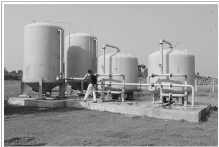
Fig. 16.9 Kola arsenic and iron removal plant
