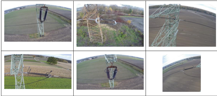
Fig. 5. Selected digital images depicting insulators on existing power lines.
