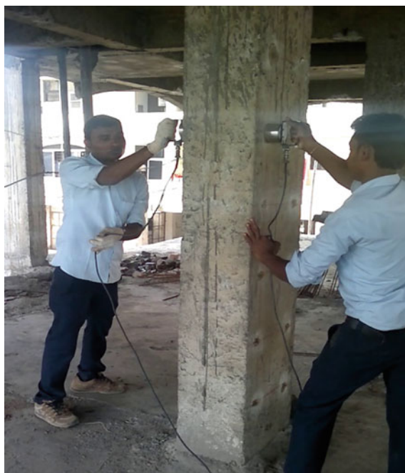
Fig. 7 Direct or cross probing method i.e. on the opposite faces of column
