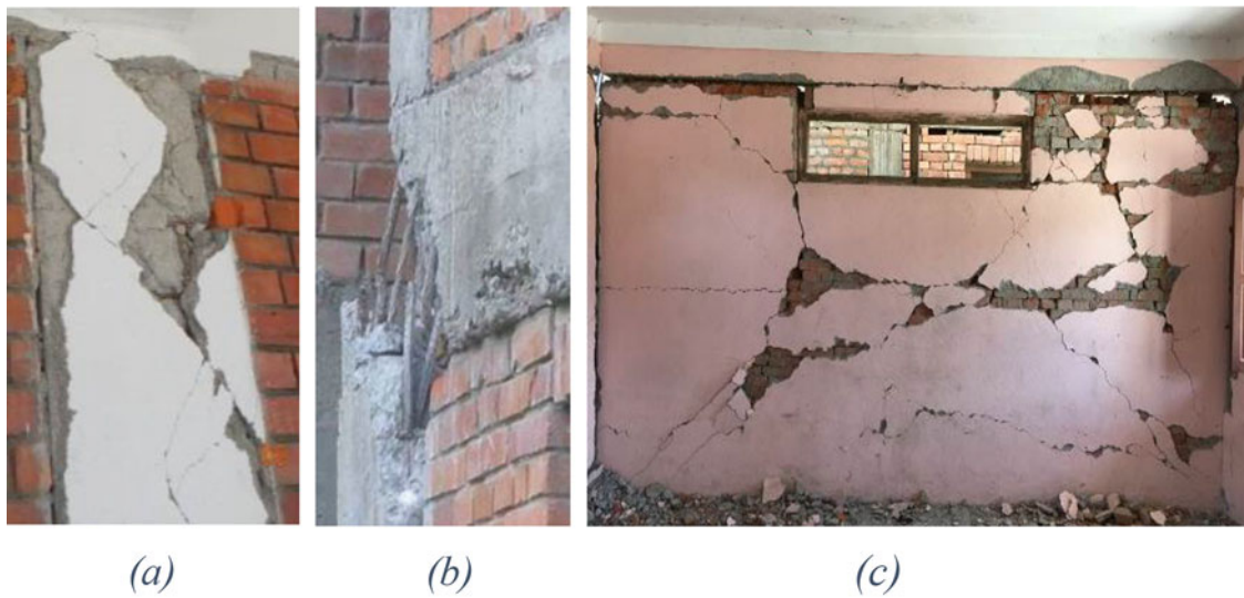
Fig. 28.2 Observed damages in the first story of the building (a) Column G2 (b) Column H1 (c) Infill wall H12
