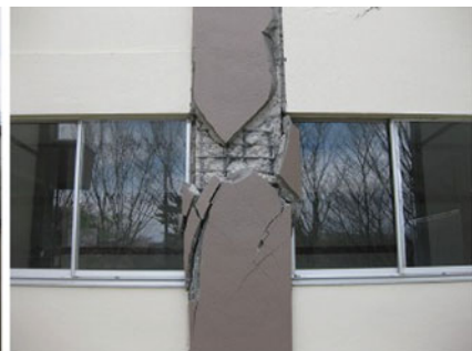
(b) Shear failure of short columns
