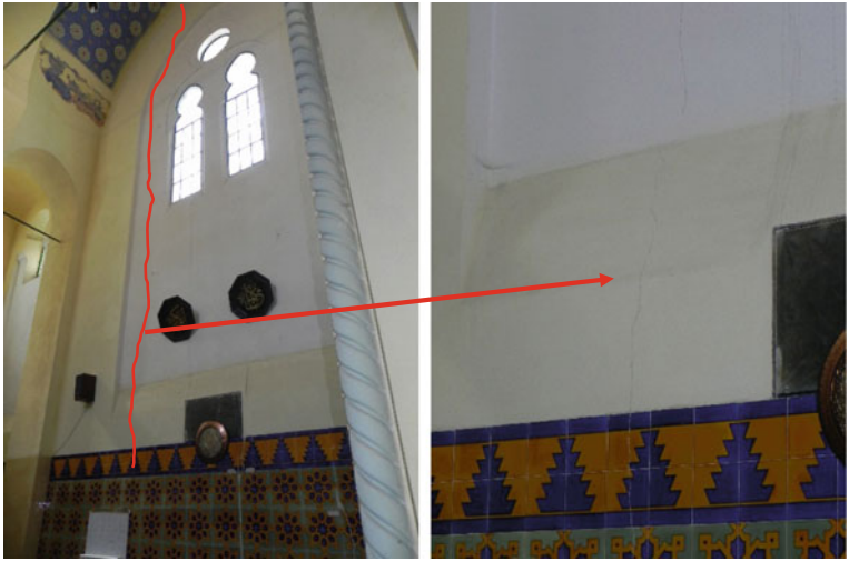
Fig. 11 Vertical cracks developed on the entire height of the masonry wall
