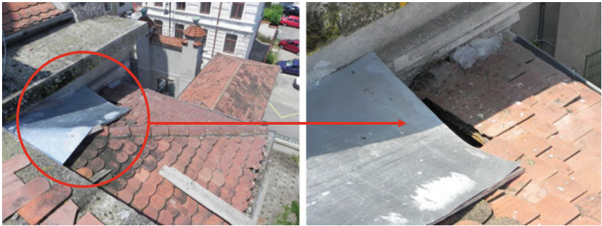
Fig. 12 Broken tiles and damaged roof in the lower part of the dome
