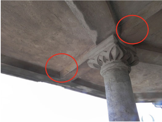
Fig. 15 Cracks in the plastering layer of the RC beams that supports the roof of the minaret balcony
