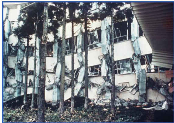
Fig. 1 Collapse of RC buildings in 1968 Tokachi-oki earthquake
