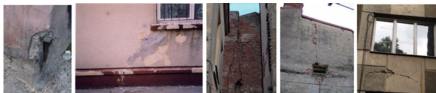
Fig. 8 Different types of structural degradations
