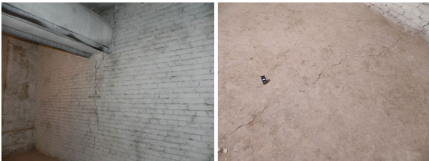
Fig. 10 Wide-opened cracks in a masonry wall in the basement and in the bare ground flooring
