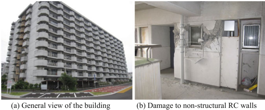
Fig. 8 Damage to a residential building in 2011 East Japan Earthquake
