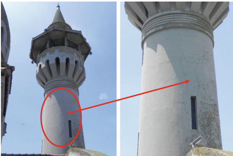
Fig. 14 Minor cracks in the exterior jacketing layer of the RC minaret of the mosque
