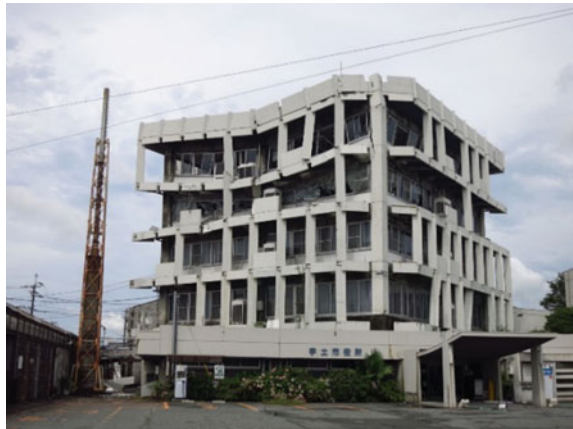
Fig. 10 Damage to city hall building in 2016 Kumamoto Earthquake
