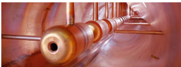
Fig. 5.18 Inside view of the Fermilab drift-tube linac. Note the vertical drift-tube supports and side-mounted post couplers that are used to stabilize the RF field in the tank ( www-bd.fnal.gov )
