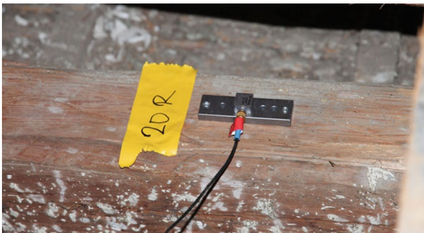
Fig. 14.13 MP 20R, cross girder mid point reference point instrumented. Special supporting steel bars have been developed to allow quick sensor roving
