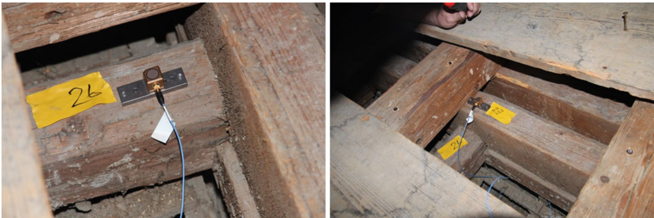
Fig. 14.14 MP 26, cross girder end point (left), and MP 27, timber truss lower chord (right), the latter consists of two beams in parallel
