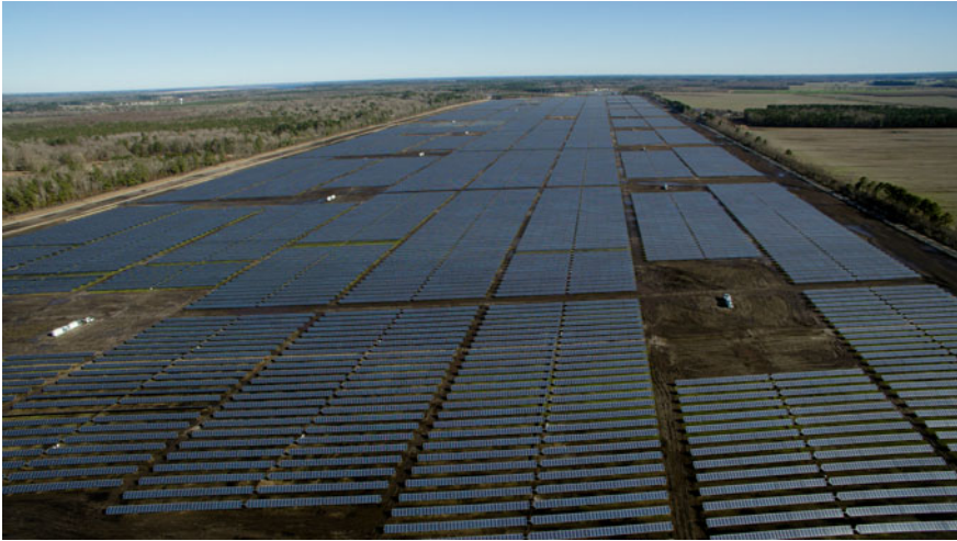
Fig. 2.2 Summit farms 60 MW solar array, North Carolina
