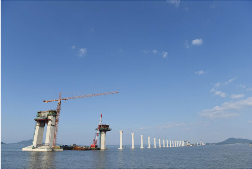
Fig. 1 New Millennium Bridge. Constructing one of biggest island-connecting bridge connecting Amtaedo Island and Aphaedo Island, Shinan-gun, Korea. Aphaedo Island already connected to Mokpo City
