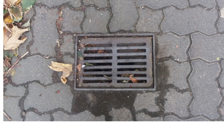
Fig. 7. A drain on the ground
