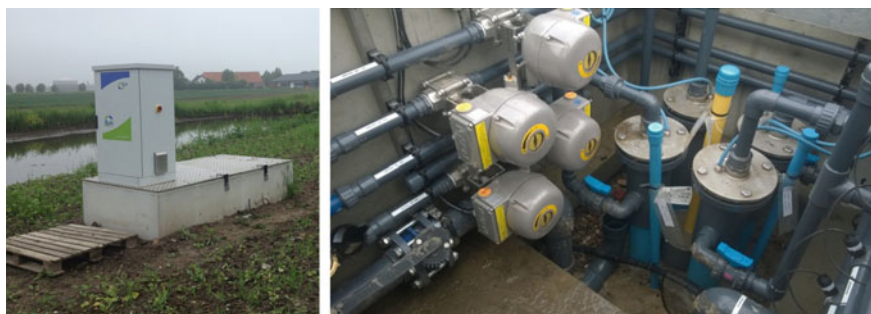
Fig. 6 The first ASR-well (PP1) in the well field in Dinteloord (left) and its well completion including control valves in the well house (right)
