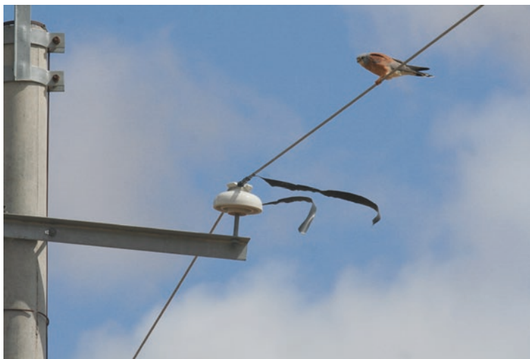
Fig. 12.9 Example of insulating tape coming loose from a retrofitted structure in the Mongolian steppe
