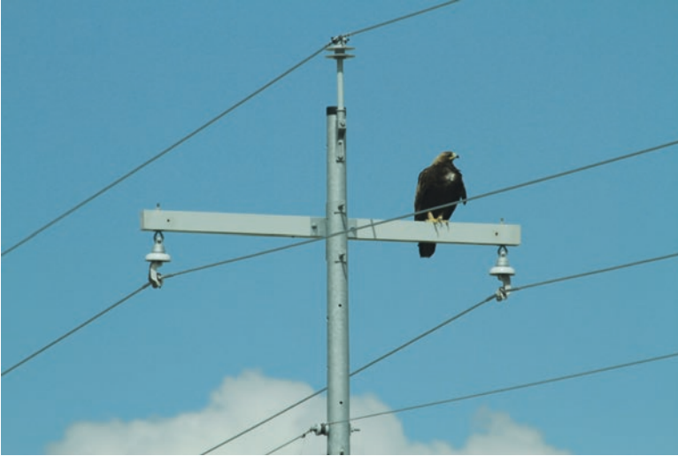
Fig. 12.6 Eagle perched on a crossarm fitted with suspended insulators
