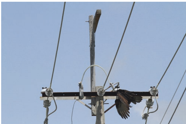
Fig. 12.1 Turkey vulture electrocution on a grounded pole with a grounded metal crossarm; note ineffective wooden elevated perch
