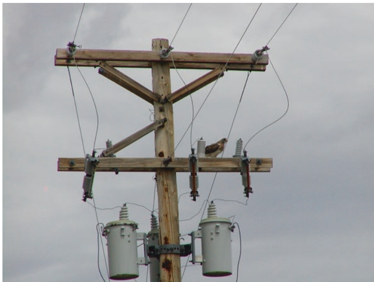
Fig. 12.3 Swainson's hawk at risk on an unprotected three-phase transformer bank
