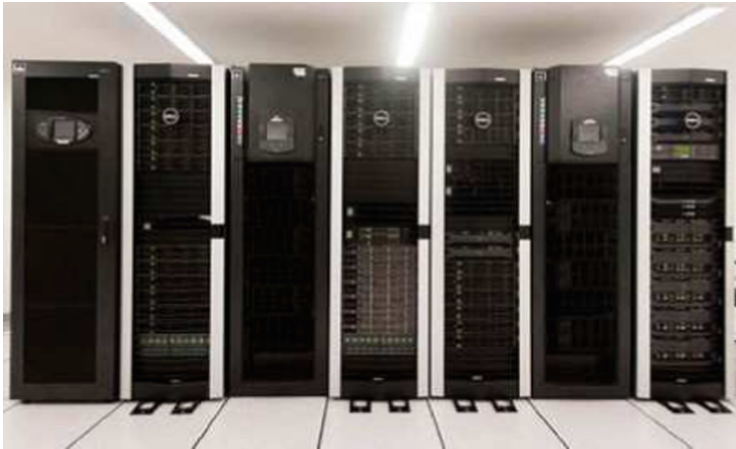
Fig. 1. TUPAC supercomputer. Seven racks hosts all the support and computing equipment, UPS and in-row water based air conditioning system.
