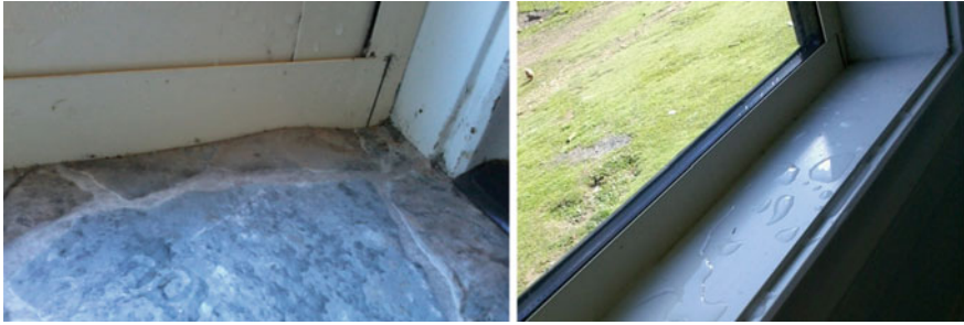
Fig. 19 Condensation forming on the kitchen flooring due to poorly installed insulation and a vapour impermeable vinyl finish. Around the window reveals the thermal bridging of the structure results in condensation
