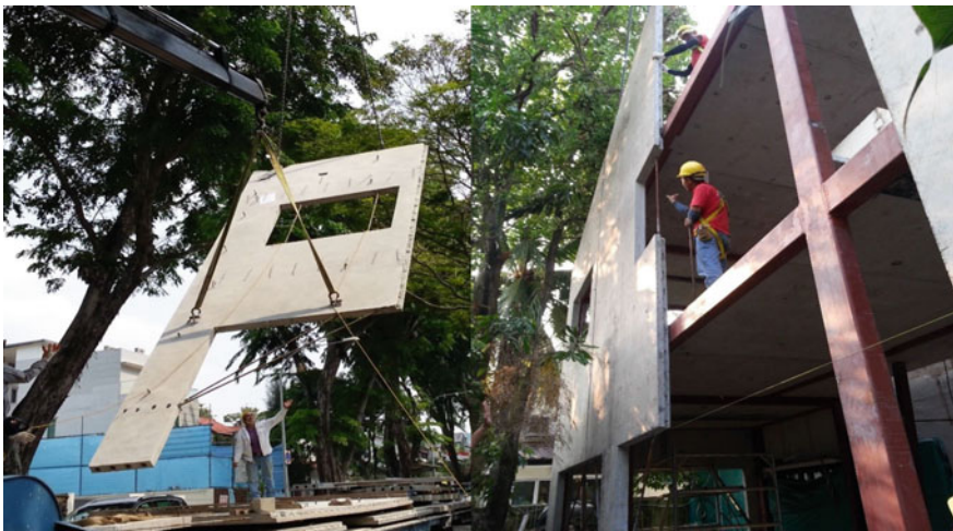
Fig. 7 Lifting of pre-cast wall and installing and clad onto modules at side elevation
