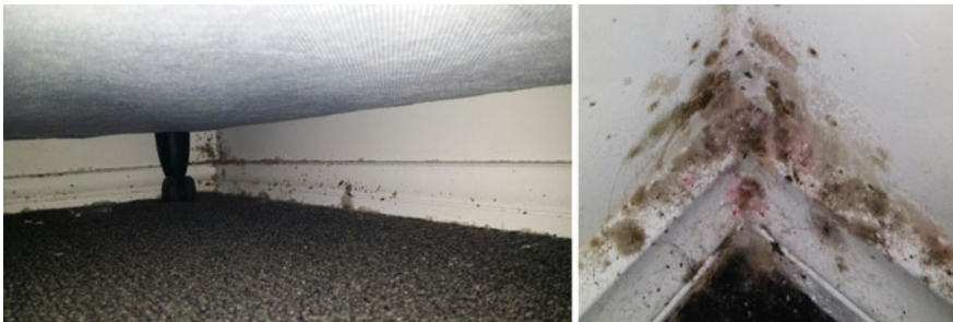
Fig. 20 Under the bed, the wall and carpet have limited exposure to the heating and experience thermal bridging to the external walls
