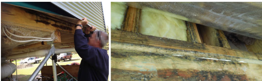
Fig. 5 Often the true effect of condensation happens inside the wall framing. A builder helps dismantle the sheet metal cladding that is hard fixed against the studs (no battens) causing the wrap to be thermally bridged with the cold exterior. Indoor vapour, unable to pass through the foil wrap condenses on the insulation which acts as a reservoir, keeping the studs and bottom plate a moist breeding ground for mould
