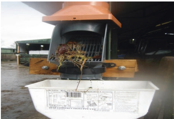
Fig. 3.42 Filter unit on downpipes
