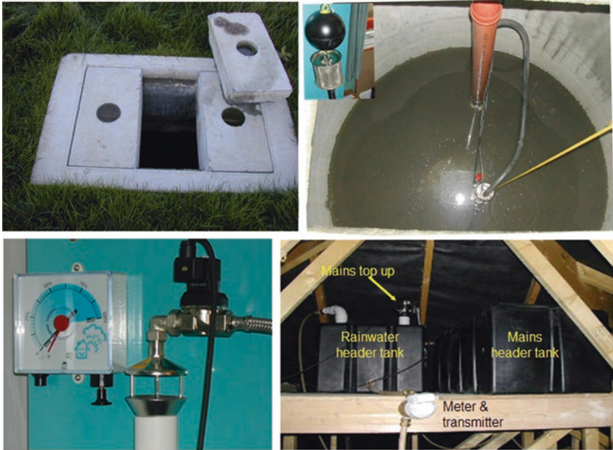
Fig. 3.40 Domestic rainwater harvesting system, Carlow
