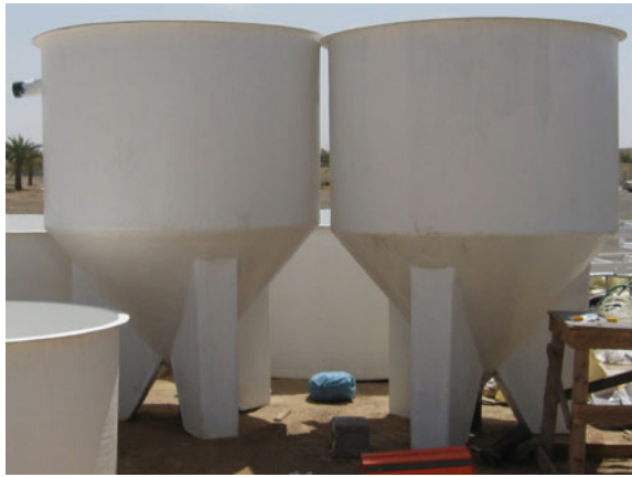
Fig. 7.13 Clarifiers with 60° conical bottoms
