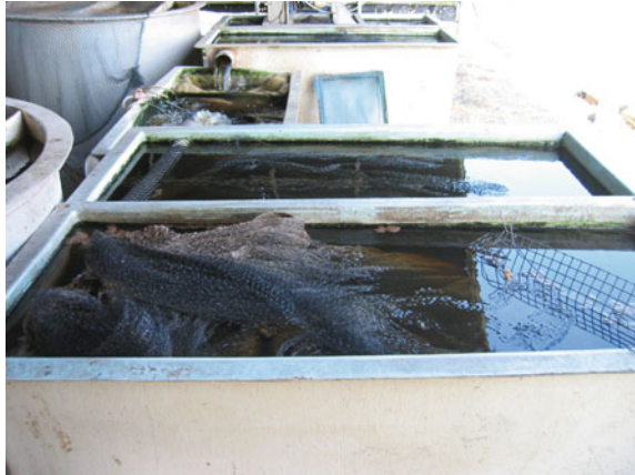
Fig. 7.14 Filter tanks to capture fine solids by means of orchard type nets
