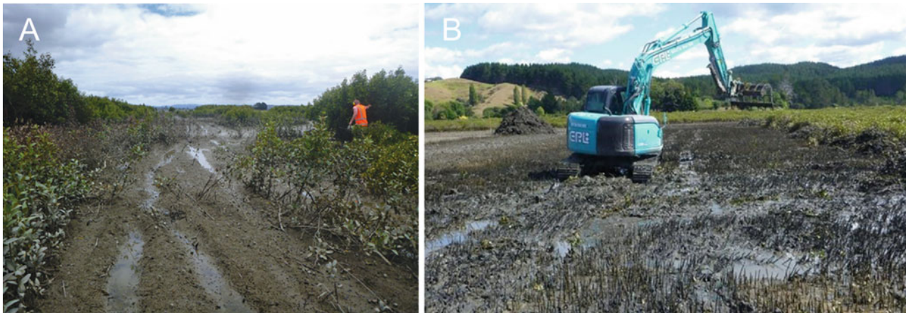
Fig. 2.13 Mangrove clearance in New Zealand: (a) manual mangrove clearance using chainsaws in Mangere Inlet, Manukau Harbour (Photo credits: C. Lundquist), and (b) mechanical clearance using digger with rake attachment at Whangamata (Photo credits: R. Bulmer)
