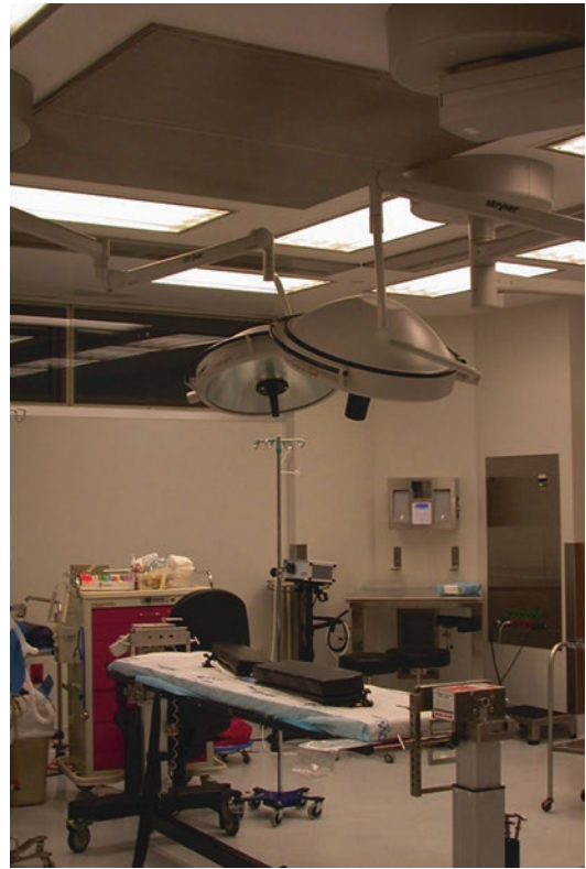
Fig. 5.6 The laminar airflow system in the roof of the operating room should be just above the operating table. The overhead lights are mounted on articulating arms in the same area
