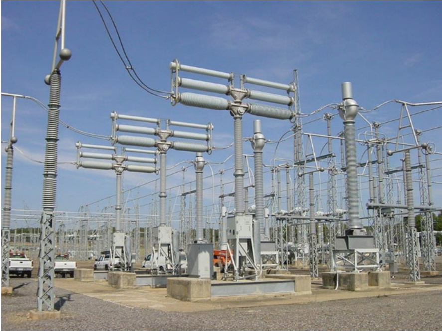
Fig. 2.32 550 kV live-tank SF 6 gas circuit breaker (Courtesy of Dominion Energy)
