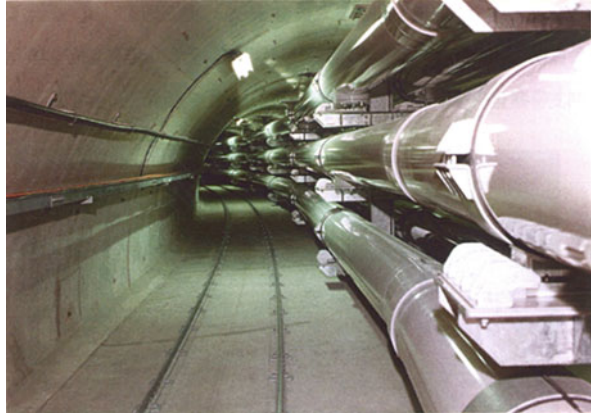
Fig. 2.17 275 kV 6300 A gas-insulated lines with length of 3 km. (Courtesy of Chubu Electric Power)
