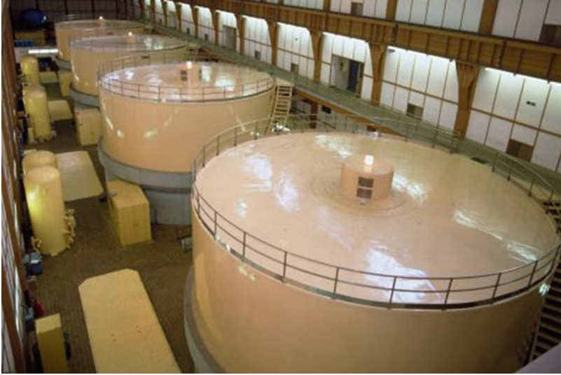
Fig. 2.5 87.5 MW salient-pole generator, 350 MW/4 units, 50/60 Hz dual frequencies. (Courtesy of J Power)
