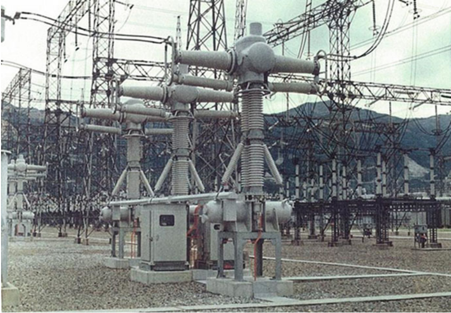
Fig. 2.30 240 kV double-pressure-type SF 6 puffer circuit breaker
