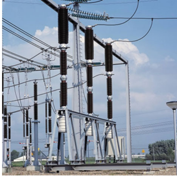
Fig. 2.10 Three single-phase independent operated gas circuit breakers. (Courtesy of TenneT TSO B.V)
