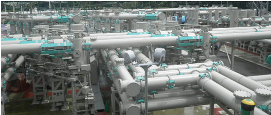
Fig. 2.16 Gas-insulated busbar in 550 kV substation (GIB). (Courtesy of Kansai Electric Power)
