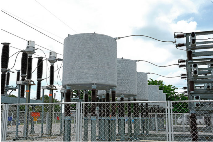
Fig. 13.6 Example of a CLR installation
