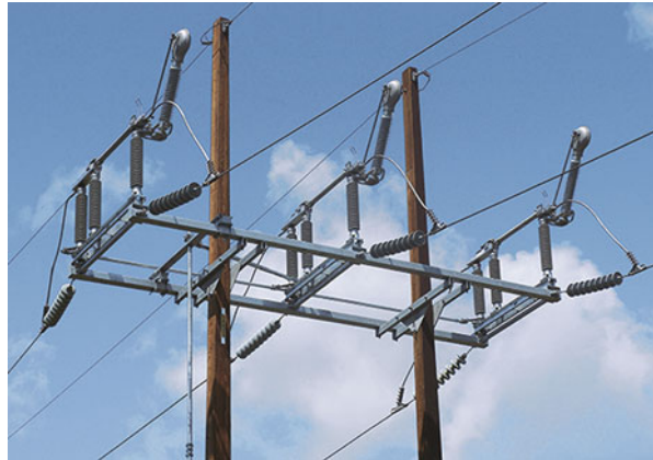
Fig. 9.21 Vertical break disconnecting switch with added SF 6 gas load break device. (Courtesy of Southern States LLC)
