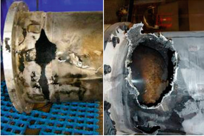
Fig. 12.7 Examples of burn through of a HV GIS enclosure
