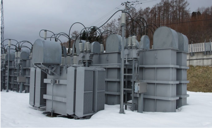
Fig. 2.23 23 kV, 22.5 MVA shunt capacitor bank. (Courtesy of J Power)
