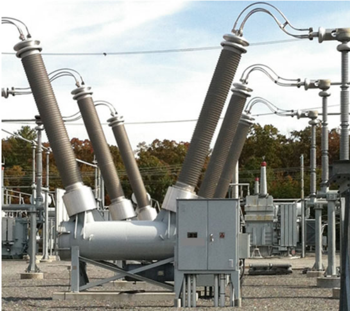
Fig. 5.27 550 kV dead tank SF 6 gas circuit breaker with a pneumatic operating mechanism. (Courtesy of Dominion Energy)
