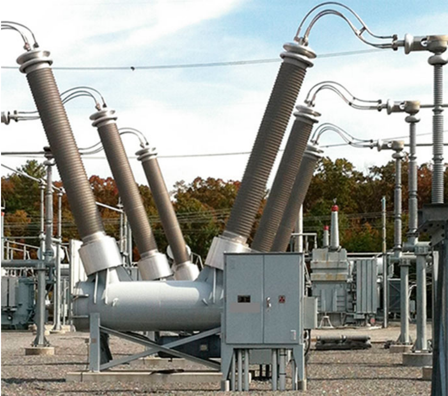
Fig. 6.14 An example of 550 kV single pressure-type dead tank gas circuit breaker. (Courtesy of Dominion Energy)
