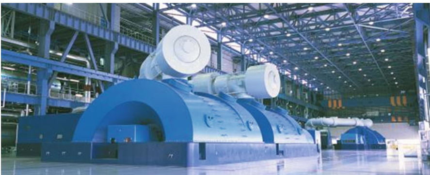
Fig. 2.4 1050 MW turbine generator, 2100 MW/2 units (Courtesy of J Power)
