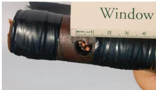
Fig. 13.13 Damage limited from a 25 kA rms, sym fault with a pyrotechnic FCL installed (Deal 2009)
