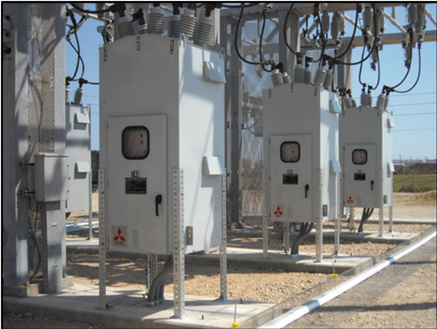
Fig. 5.35 Example of outdoor vacuum circuit breaker. (Courtesy of Mitsubishi Electric Power Products)
