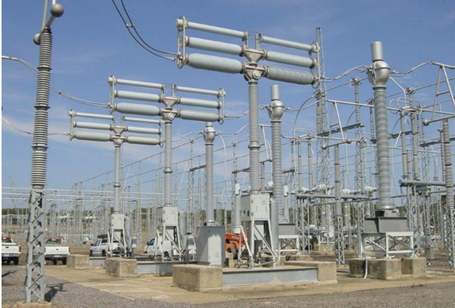
Fig. 5.26 550 kV live tank SF 6 gas circuit breaker. (Courtesy of Dominion Energy)
