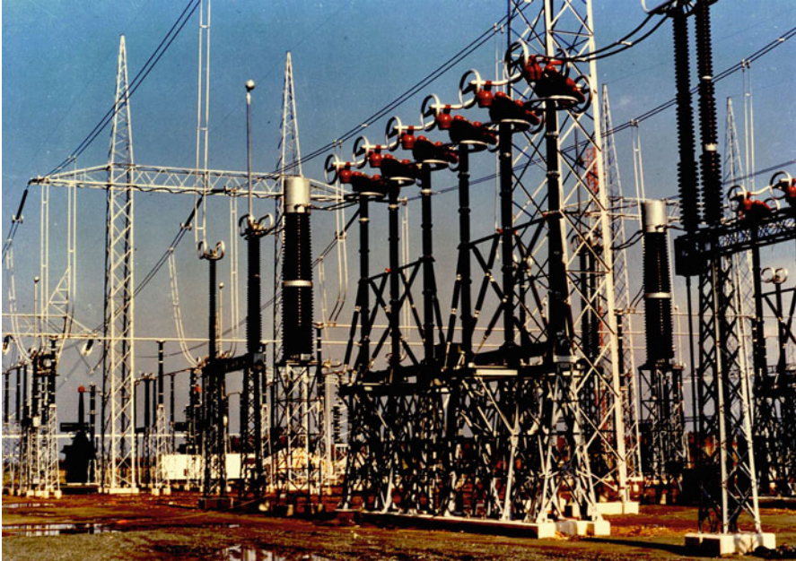
Fig. 2.29 Latest-generation 800 kV air-blast circuit breaker. (Courtesy of GE, produced by Alstom)
