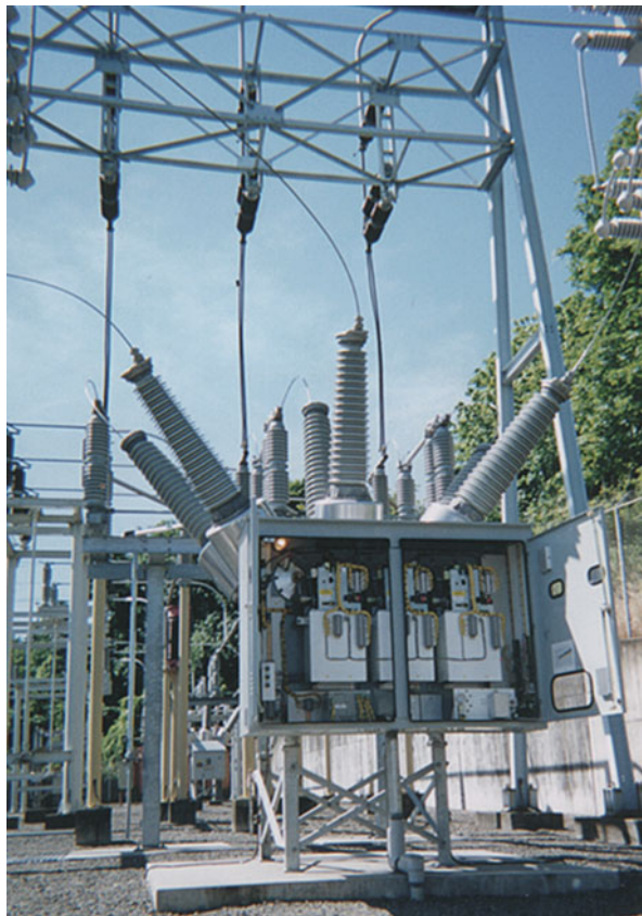
Fig. 14.37 CSS applied to 121 kV capacitor bank
