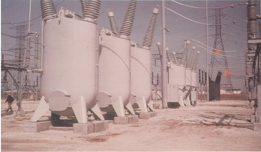
Fig. 5.19 345 kV 63 kA oil circuit breakers
