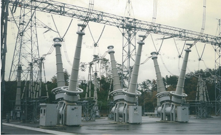
Fig. 5.28 550 kV single pressure-type gas circuit breaker. (Courtesy of Chugoku Electric Power)
