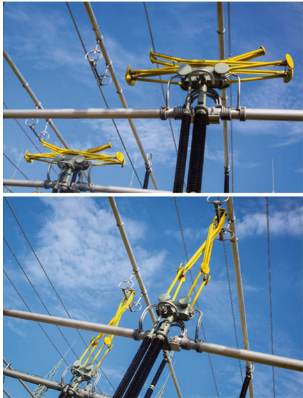
Fig. 9.17 Pantograph-type disconnecting switch. (Courtesy of Hapam B.V.)
