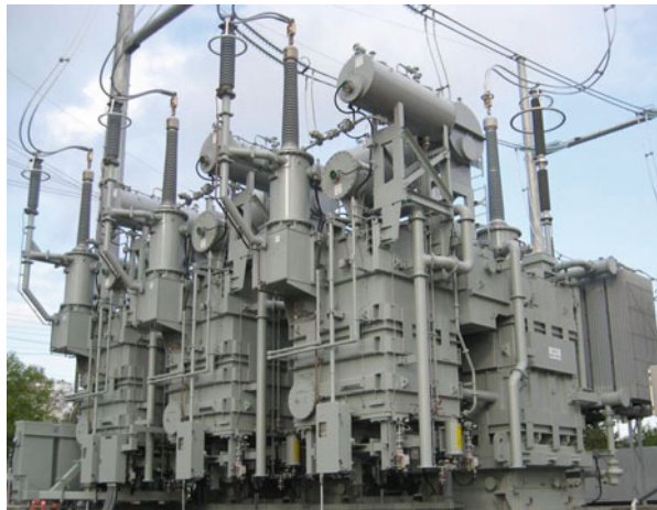
Fig. 2.21 345 kV 750 MVA power transformer (shell type)
