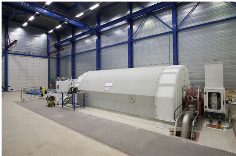
Fig. 11.2 2200 MVA short-circuit generator in order to enable high-power testing with short-circuit current of variable power frequency. (Courtesy of DNV GL, KEMA Laboratories)
