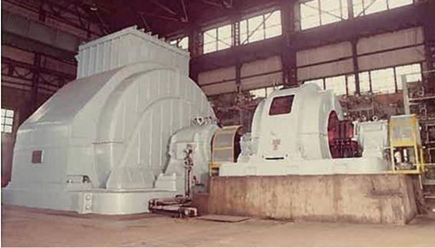
Fig. 11.3 50 MVA 13.2 kV vintage short-circuit generator
