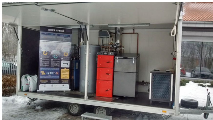
Fig. 1 The “PoLoNEs” mobile installation
