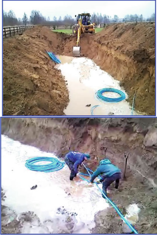
Fig. 2 Laying the ground source heat pump system at a depth of 1.9 m, 10 loops 100 m each, active area of the exchanger is 11 m × 23 m (photo by authors)
