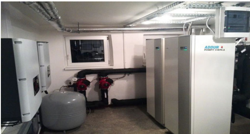
Fig. 2 View of the system engine room located in Szczytno. Source Addur
