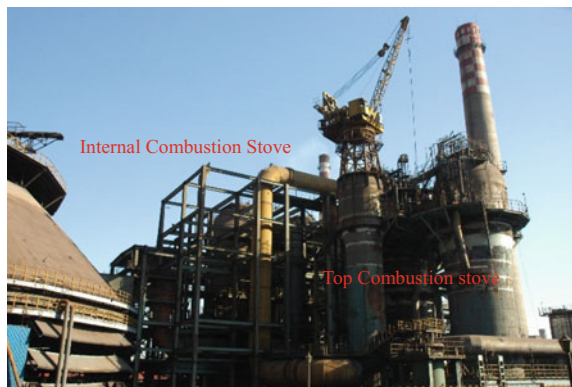
Fig. 2 Photo of Shougang's No. 2 BF hot blast stove
