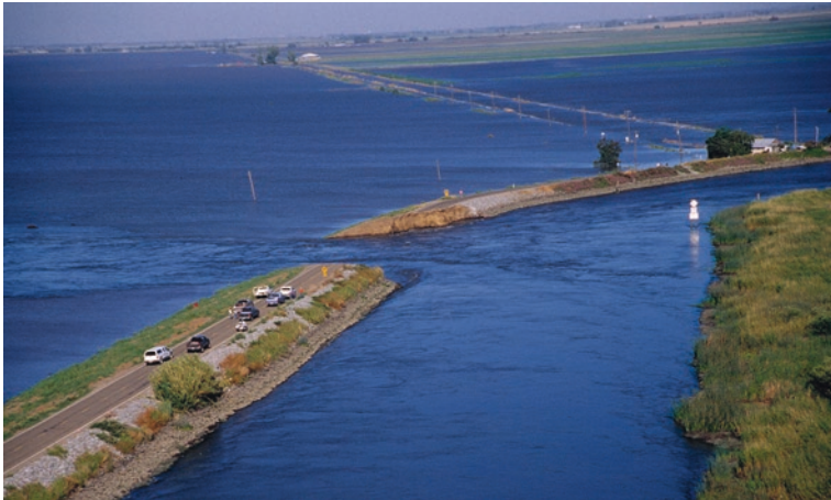
Fig. 3.2 Jones Tract levee failure in June 2004, California (Courtesy of California Department of Water Resources)
