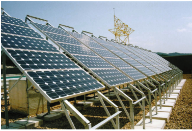
(a) SUNSET PV solar power system in Zamudio (Spain).
