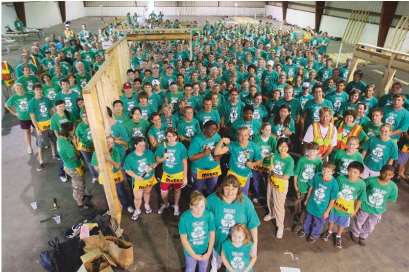
Fig. 3.6 Freshman class prefabricates walls of home for Habitat for Humanity International, 2007. Photo by Mark Schiefelbein
