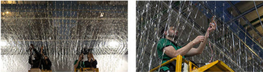
Fig. 3.9 a Case study 2, suspended structure. b (Left) Participatory process, the students taught workers the fabrication method. (Right) Worker participating into the fabrication process (Photos by Deborah Lopez, Hadin Charbel, Obuchi Lab)
