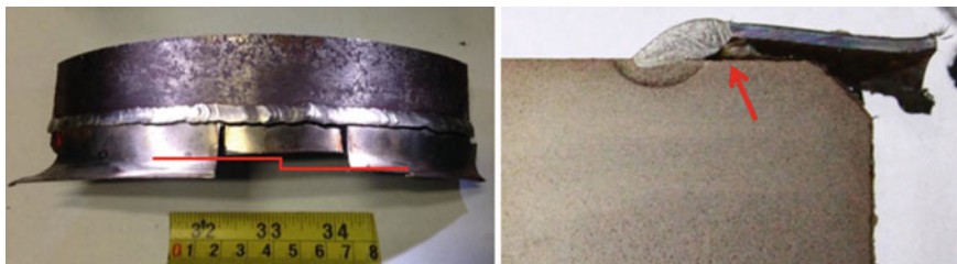
Fig. 5 Cross section of the fracture zone (The arrow points to the line of the fracture)
