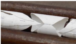
Photo 4. PVC pipe failure
