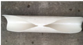
Photo 7. PVC pipe failure
