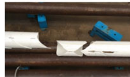
Photo 6. PVC pipe failure
