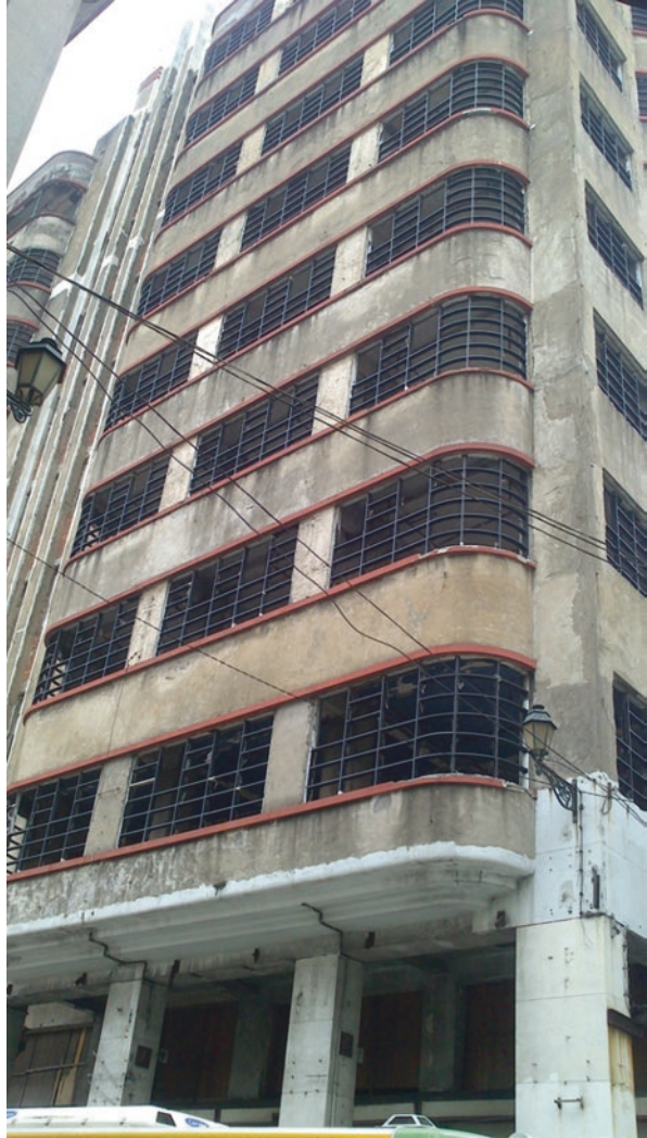
Fig. 7 The gutted dilapidated Grand Hotel
